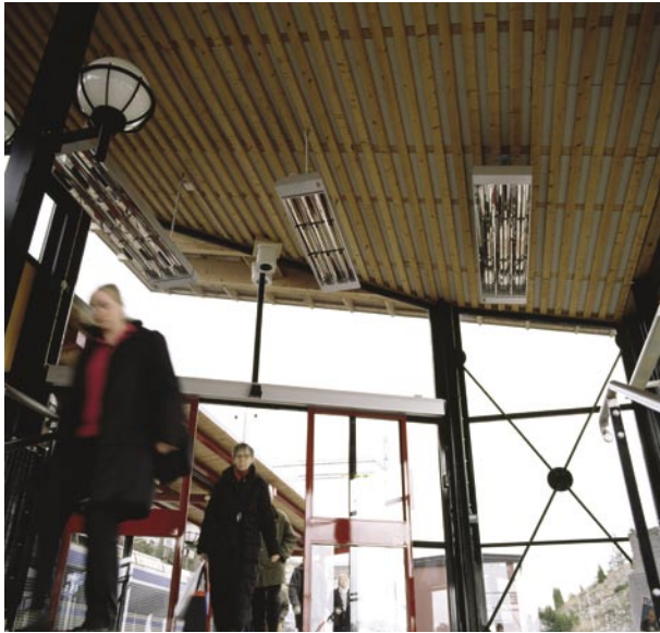
This train station outside Stockholm is heated by industrial infrared heaters. A regulator with timer allow waiting passengers to increase the heat when it is particularly cold.
